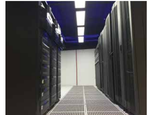
The IT server room at the National Archives. © National Archives.
